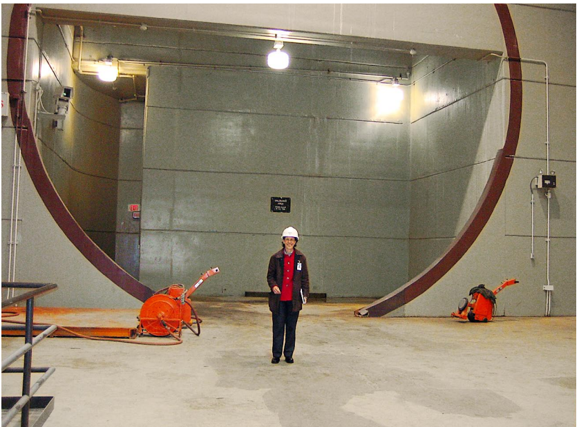
Here I am more than 300 feet underground touring the District's Mainstream Pumping Station. The large circle behind me is the size of the largest portions of Deep Tunnel.
